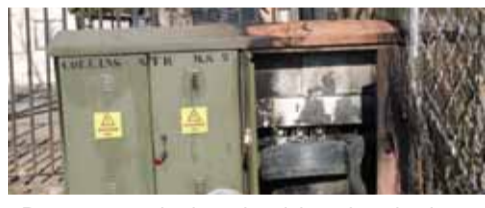
Protestors torched an electricity substation in Collins Street.
